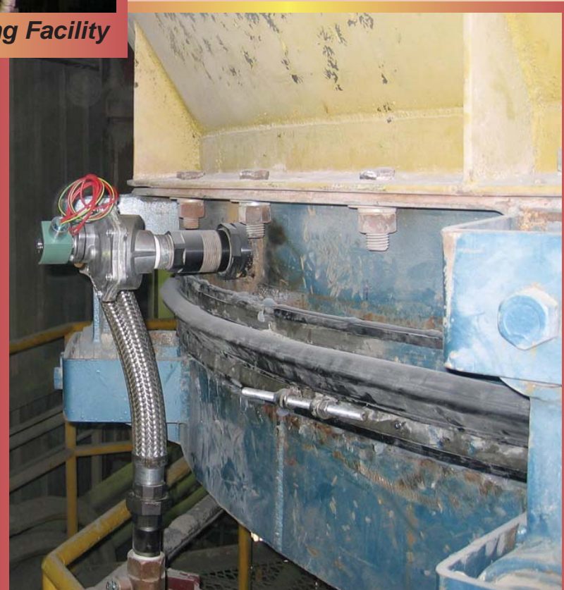
Reground Gypsum Board Processing Facility
